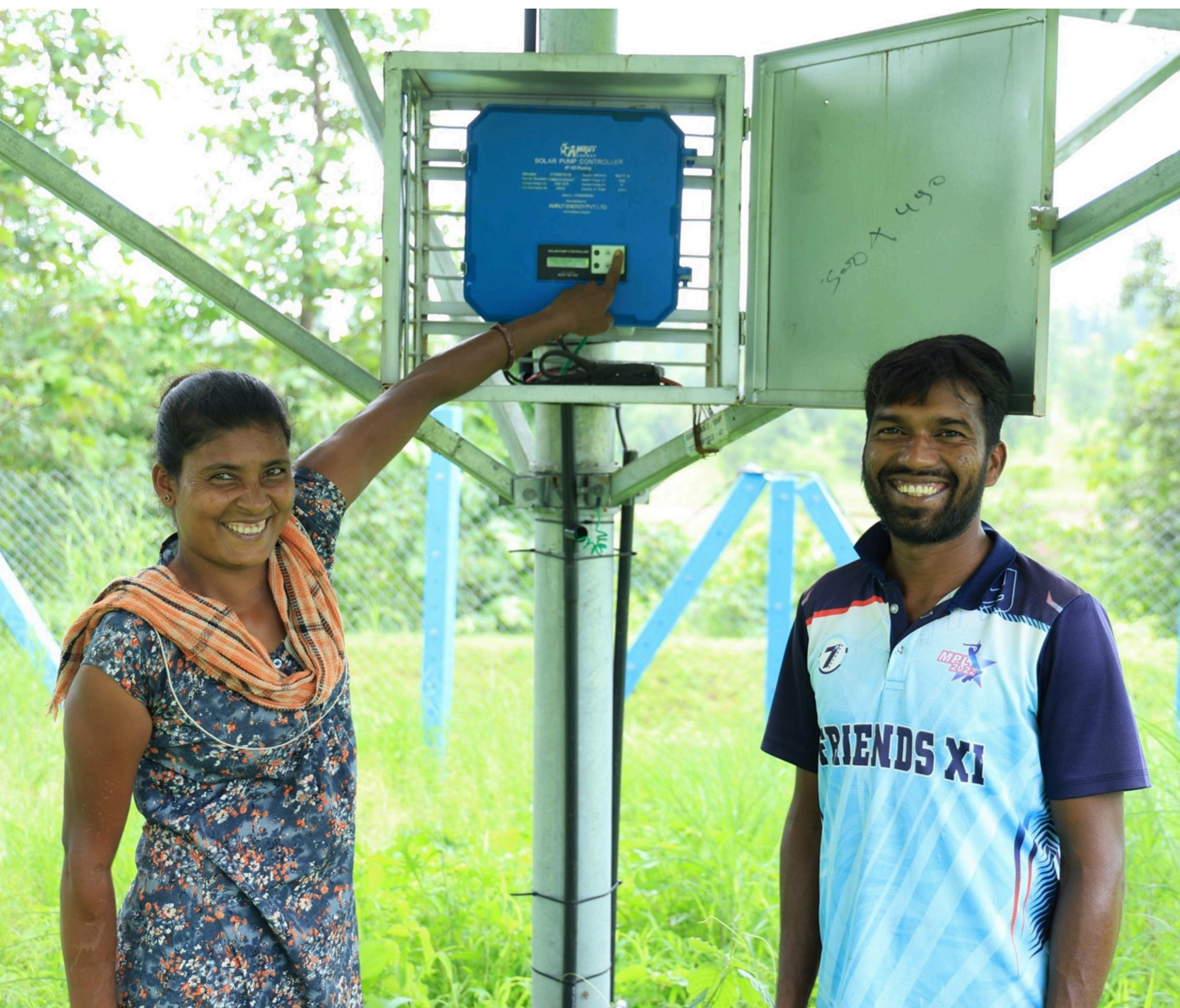
Community managed solar lift irrigation system in Subir
